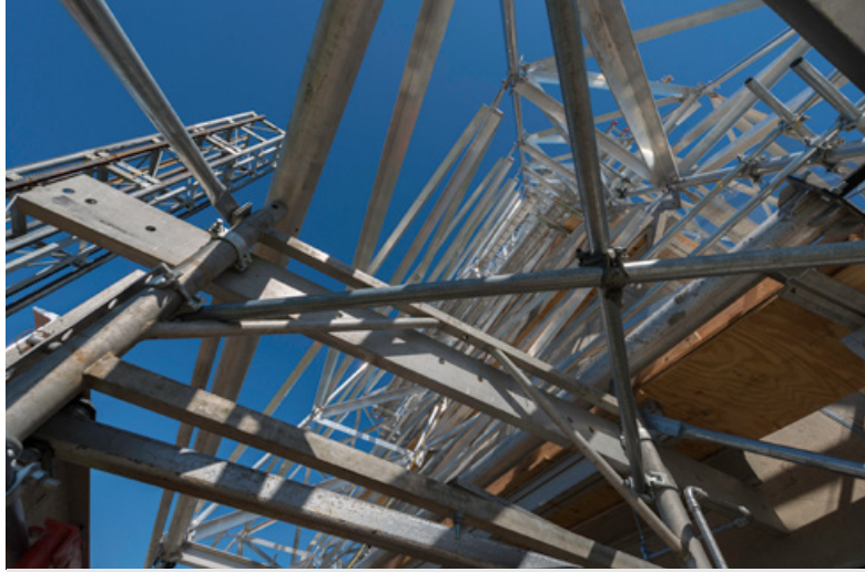
Looking upward through the scaffold at the Pyramidion shows how the crown’s structure differs from the lower structure.
