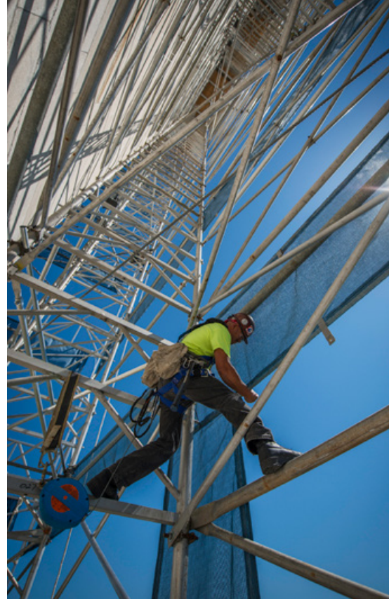
The scaffold has a 1° taper created by tilting it inward towards the monument and its end tower panels towards the center.
