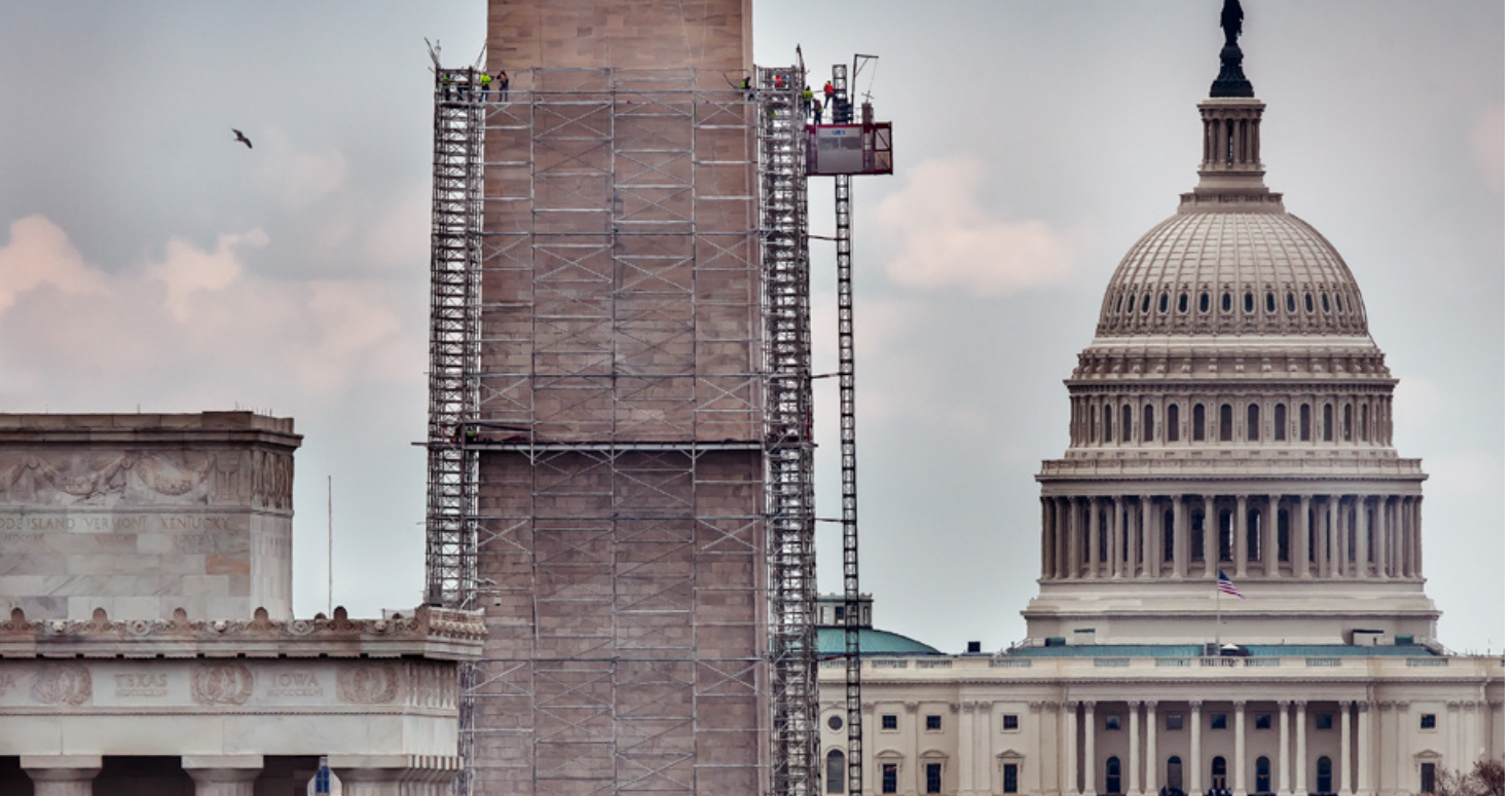
The 2013 scaffold system has the hoist, which is anchored to the scaffold, outboard of the system. In 1998 the hoist was inside the scaffold, making it difficult to access the south face.
