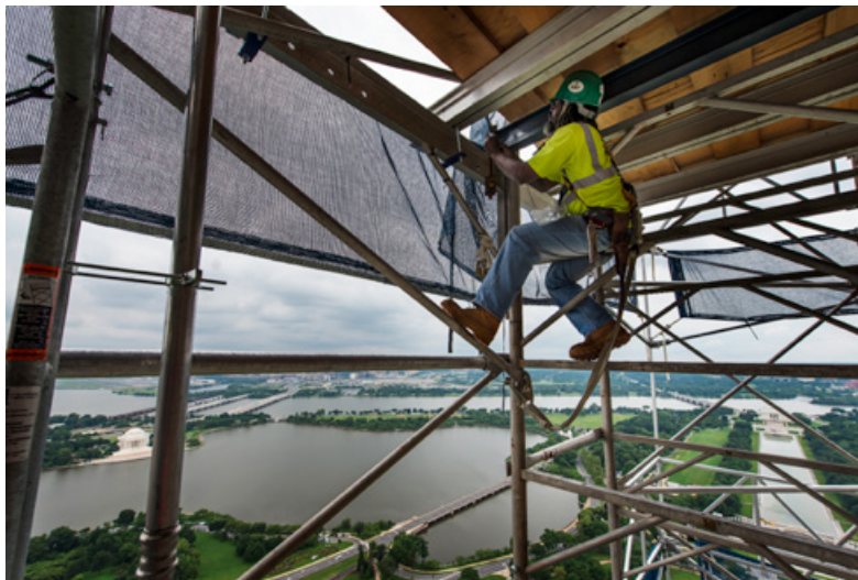
A UBS team of as little as 12 and as many as 30 met the challenge of erecting the scaffold system.
